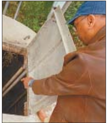
Owens pointed toward the bottom of the sewage-filled basin at 37th and Market streets in Alorton.
